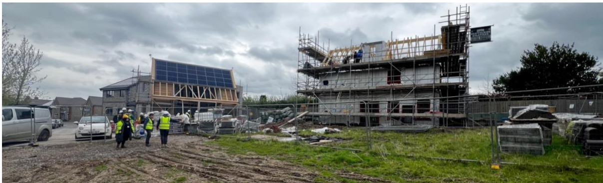
FIGURE 1: TWO PLOTS YET TO BREAK GROUND IN THE FOREGROUND, TWO SELF BUILD HOMES GOING UP AND ONE COMPLETED.
