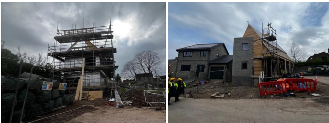
FIGURE 5: THREE OF THE SELF BUILD HOMES. THE STONE FACING OF ONE REFLECTS THE DESIGNS ON THE WIDER DEVELOPMENT
